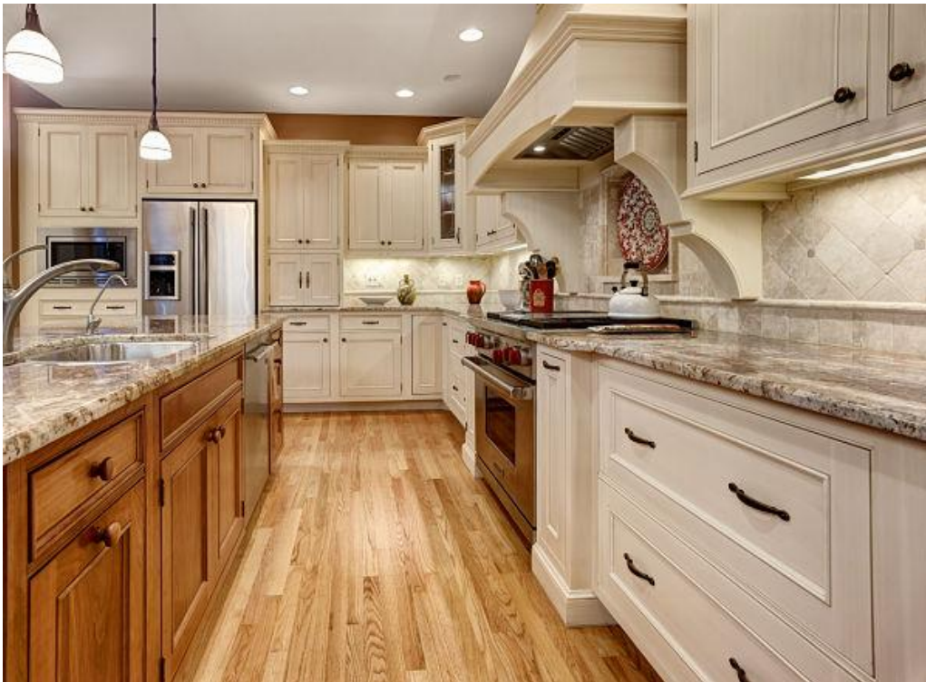
Task lighting over stove and counter areas.
